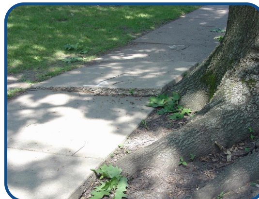
Tree roots uplifting sections of sidewalk. Such infrastructure damage can be costly and dangerous, causing pedestrians to trip and fall.
